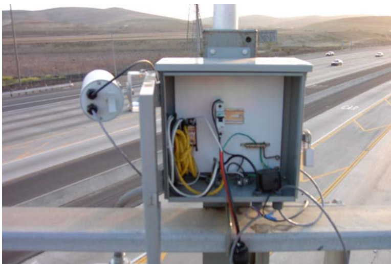
Figure 7.1. Camera electrical box.
