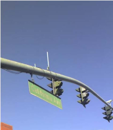
DSRC Antenna at El Camino Real and California Ave.
